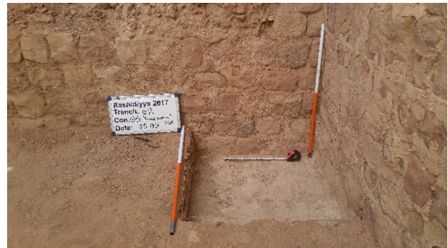
Fig. 7. The fort of Rashidiyya: the Pietra-rasa plastering on the ashlar façade, excavated from the south rampart. Source: Ayorloo, 2017, 2018.
