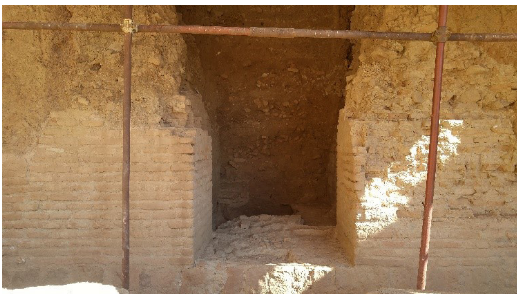
Fig. 9. A photo depicts the small S. doorway, to the right of the huge S. outwork, and the technique of skirting by Pietra-Rasa plastering and rough-hewn. Source: Ajourloo, 2018.
